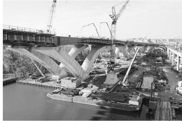
Figure 5. The complexity of megaproject construction demands disciplined communication (© 2005 David Sailors, with permission)
