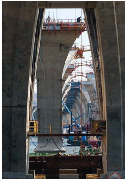
Pyramid-like foundation footings were built from 2001 to 2003 to support the bridge's V-shaped piers. Photo by David Sailors.
