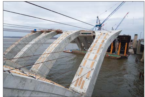
About $1 million in construction value is put in place daily at the Woodrow Wilson Bridge project. Photo by David Sailors.
